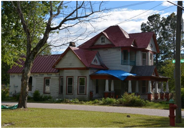
The c. 1910 John D. Finch house, purchased by Scott and MaryBeth Carpenter, is undergoing renovations, including stamped-metal shingle preservation, porch reconstruction, and a rear addition to replace extensive rot over a previously covered back porch.
